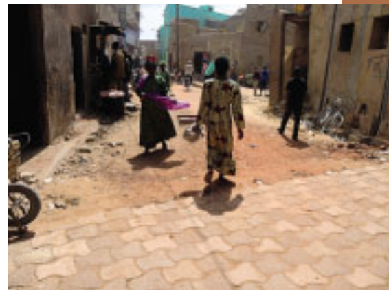
The streets are being paved with bricks made from recycled local refuse, such as plastic bags.
