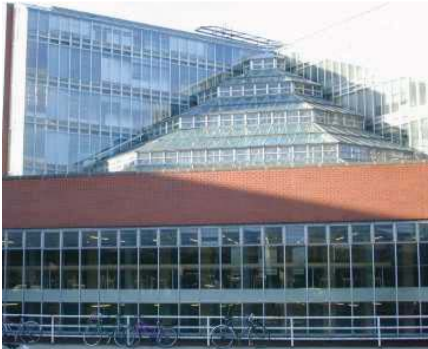
Figure 6: Built in the 1960s, a time when environmental concerns played little or no part in the design of buildings, the Cambridge University History Faculty was effectively a giant glasshouse – more than enough daylight, but too hot in summer, too cold in winter. Paradoxically the building was awarded a Gold Medal by the RIBA in 1966 (Source: webmaster@hist.cam.ac.uk).
