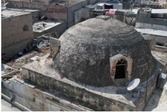
Figure 2: Dilapidation of Hammām al Kebīr; View of the Remaining Dome (Source: Authors, 2008).
