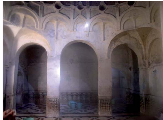
Figure 10: Warm Room of Mukhfiyya Hammām in the Medina of Fez (Photo by Jean Bouillot – November 2006).
