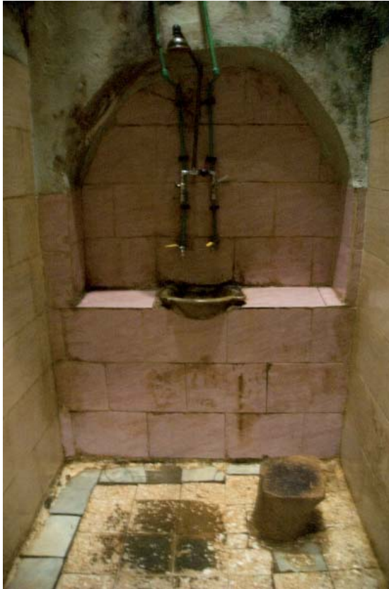
Figure 5 Inadequate Changes Inside the Bathing Spaces of the Hammām. (Source: Sibley, M- AHRC funded project: Historic Hammāms of North Africa@June 2007).
