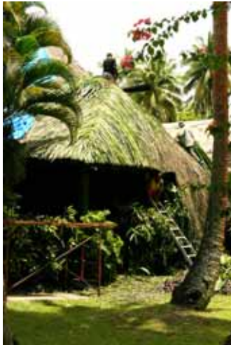
Figure 1: Repairs on a traditional Fijian roof of the dining hall, Vanua Levu resort.
