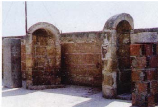
Figure 7: Cool wind catcher on the roof (Source: Authors).
